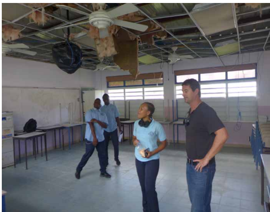
Students involved in damage assessment of their school.
